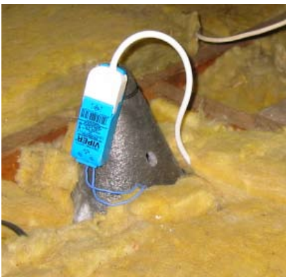
Electronic transformer installed with Basic Mitt
